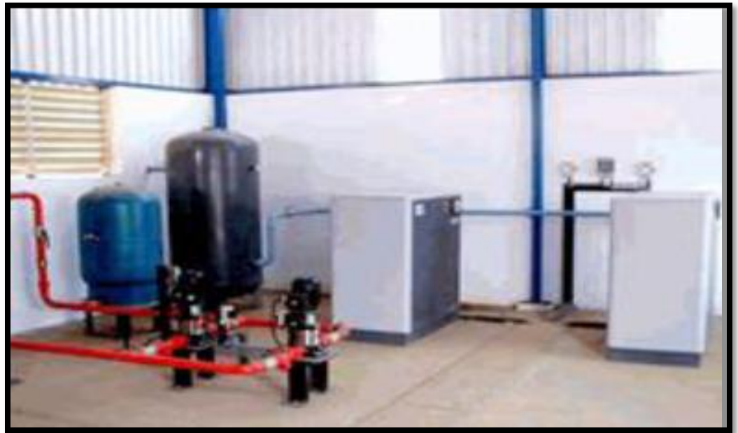
Compressed Air System
